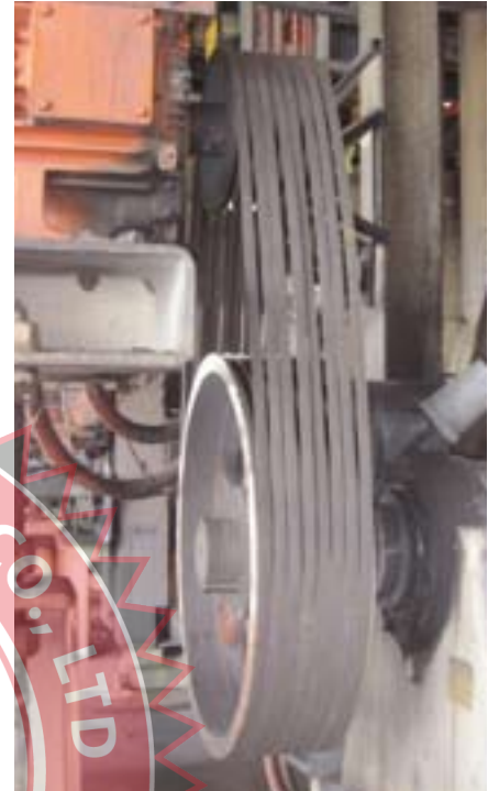
● Original V-belt Drive
